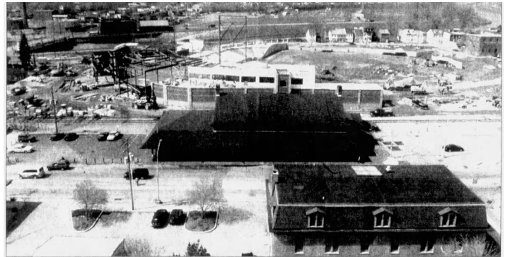
Sovereign Bank Stadium in York begins to look more like a baseball stadium, in this photo taken last Thursday. But there is still much work to be done at the construction site, and York Revolution officials announced Monday that the first home game at the new stadium will not be played until June 15.
